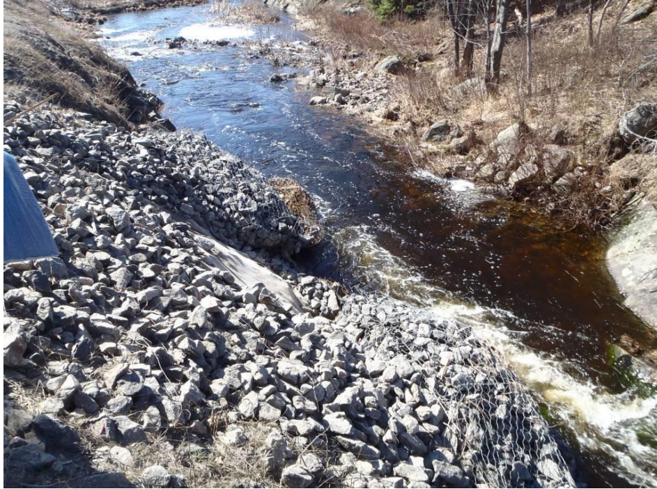
Figure 35. Slumping gabion baskets and exposed landscape fabric (looking downstream)
