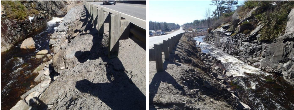
Figure 8. Erosion and runoff points into Sucker Creek between stations 1 and 2
