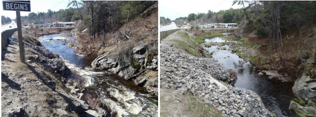
Figure 20. Sucker Creek spawning bed looking downstream. The photo on the left was taken on April 17, 2016 and the photo on the right was taken on May 12, 2016.
