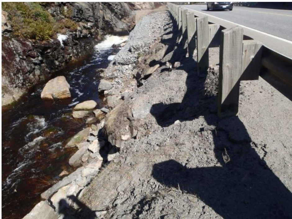
Figure 34. Areas of erosion between the highway and Sucker Creek (looking upstream)
